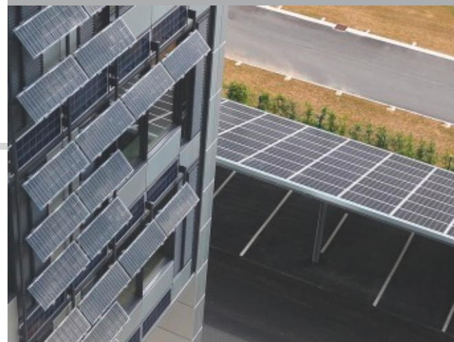
Meudon, Green Office, Bouygues Modules brise-soleil Modules: 280 LSG-70 W p Dimensions: 450 x 1.314 mm Performance: 19,6 kW p
